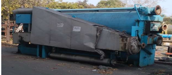
13. SCRAP IDLE ASSET - VAPOUR ABSORPTION MACHINE
